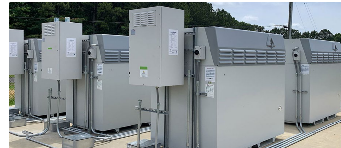
1.8MWh Flow Cell Battery – Q1 2022
